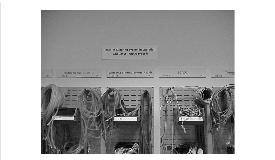
Figure 26.7: Blue bins and hanging cables at Eircom
