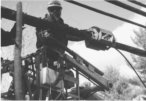
FIGURE 4.4 Typical installation of lashed aerial fiber cable.
