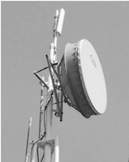
Figure 6.23 Photo of a parabolic reflector ‘dish’ antenna with shroud and radome.
