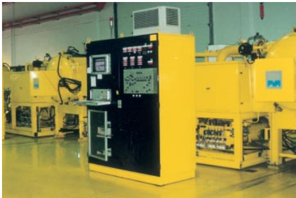
Fig. 4.1-22 Batch-batch type sintering furnace and control panel
