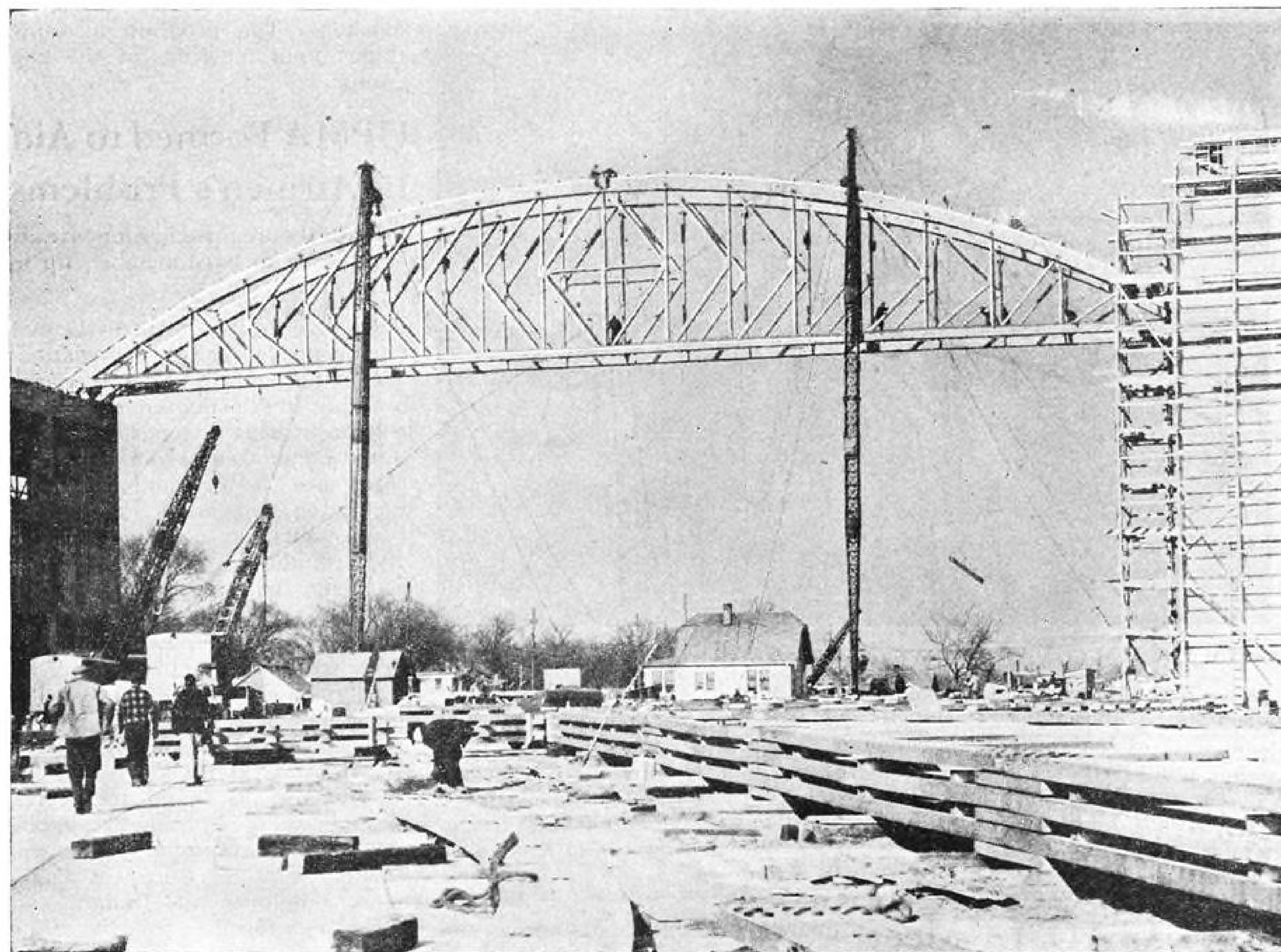
NAVAL RESEARCH HANGAR. For this hangar (260' x 110') Timber Structures fabricated 226' glued laminated bowstring trusses (world's largest). Hangar designed by Bureau of Yards and Docks. Contractor: Standard Construction Company.
