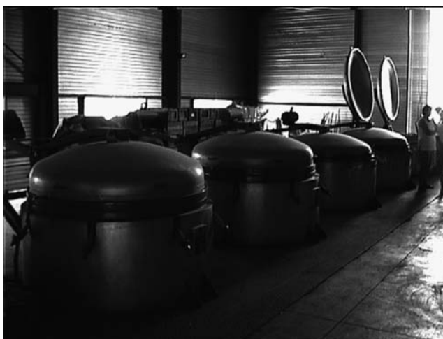
FIGURE 4.11 Battery of four distillation units.
