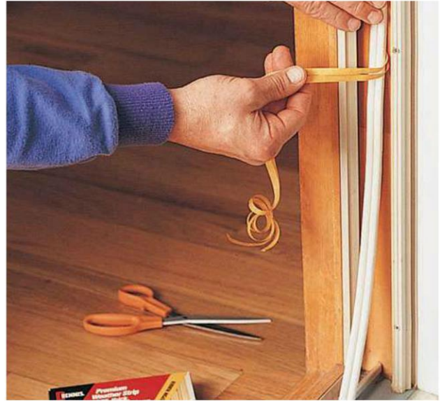
Door weatherstripping products are used to create a smoke-proof seal on the interior door leading into the cigar lounge.
